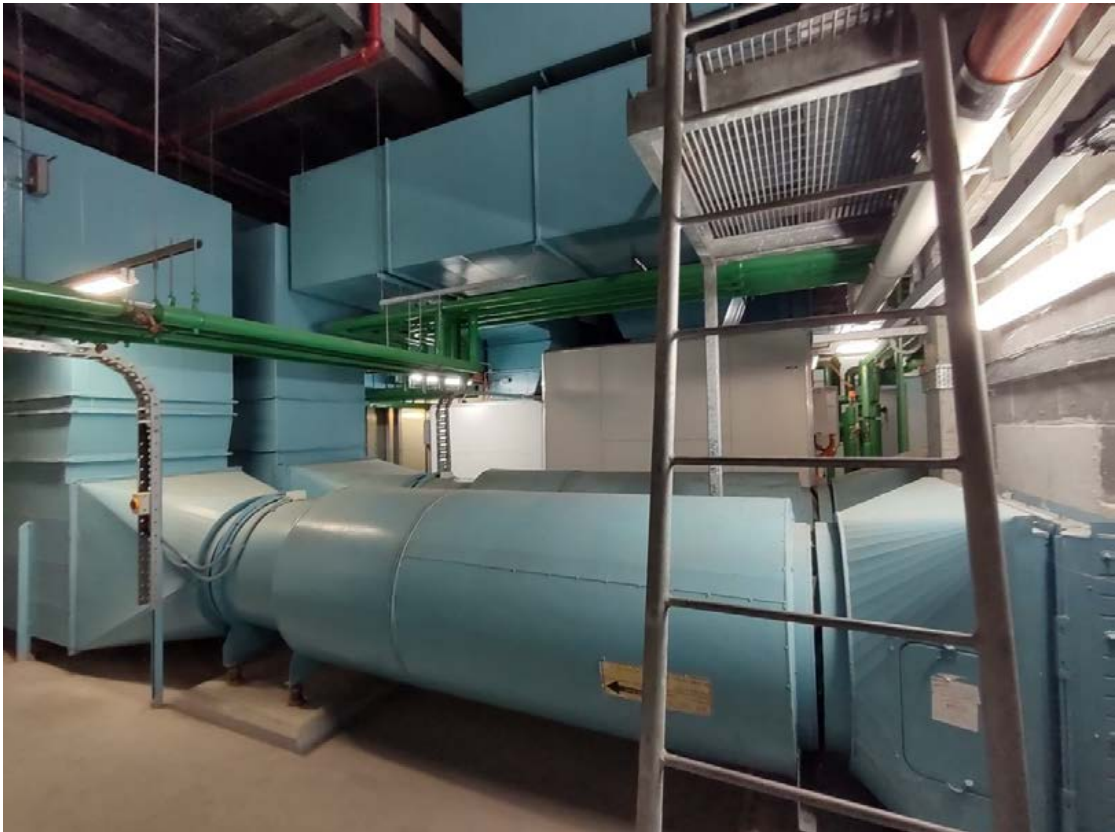
Photo 2: Plant room in level 7
