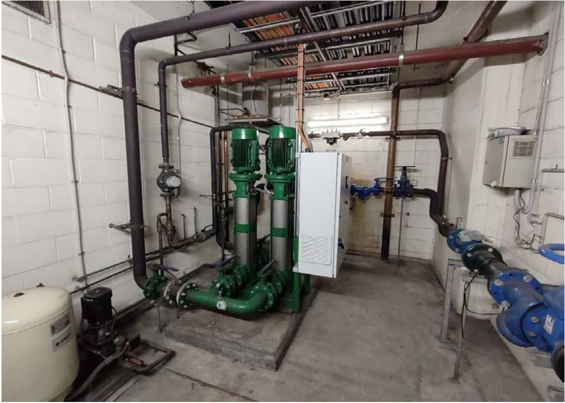
Photo 19: Water pump room in basement 2
