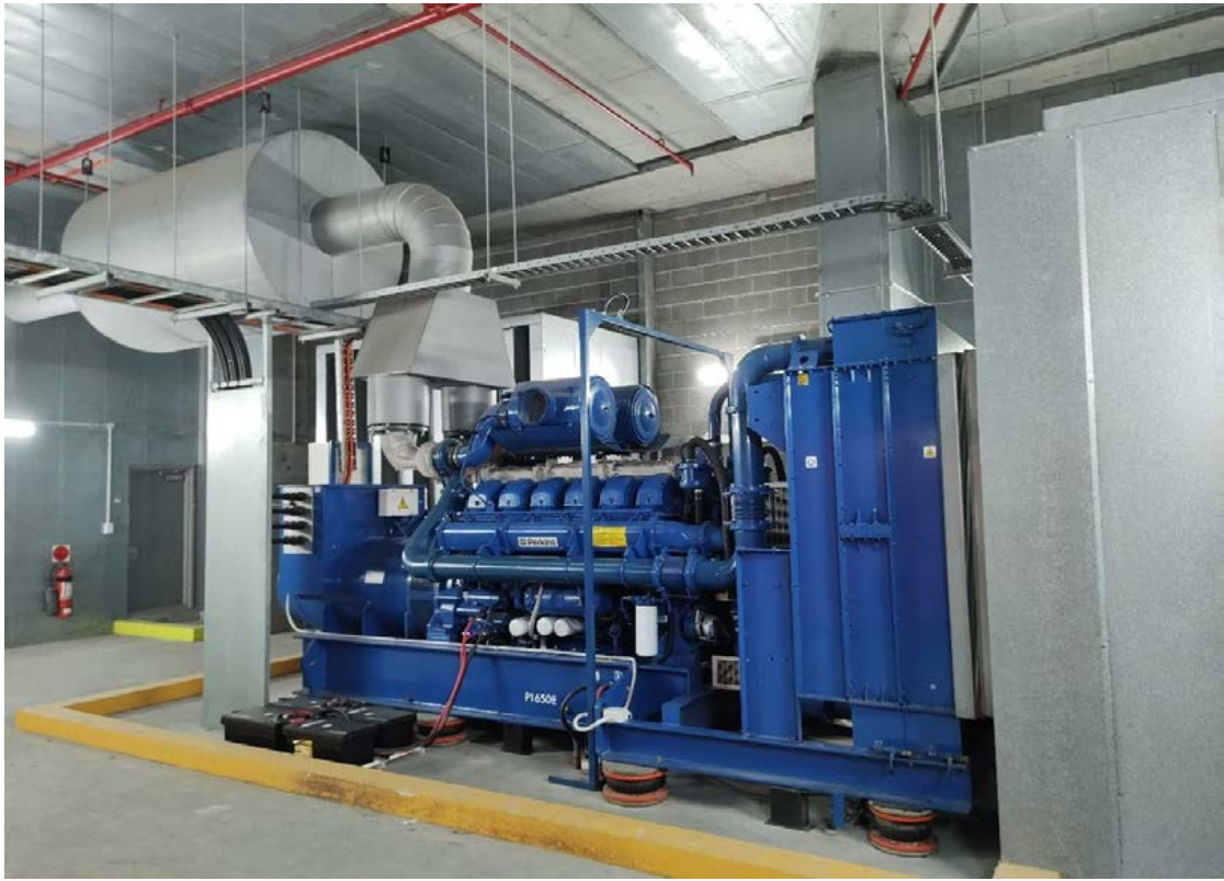
Photo 11: Diesel generator room in level 7
