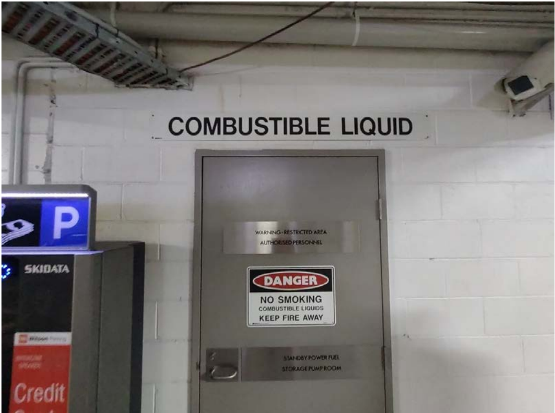
Photo 4: Standby power fuel storage pump room
