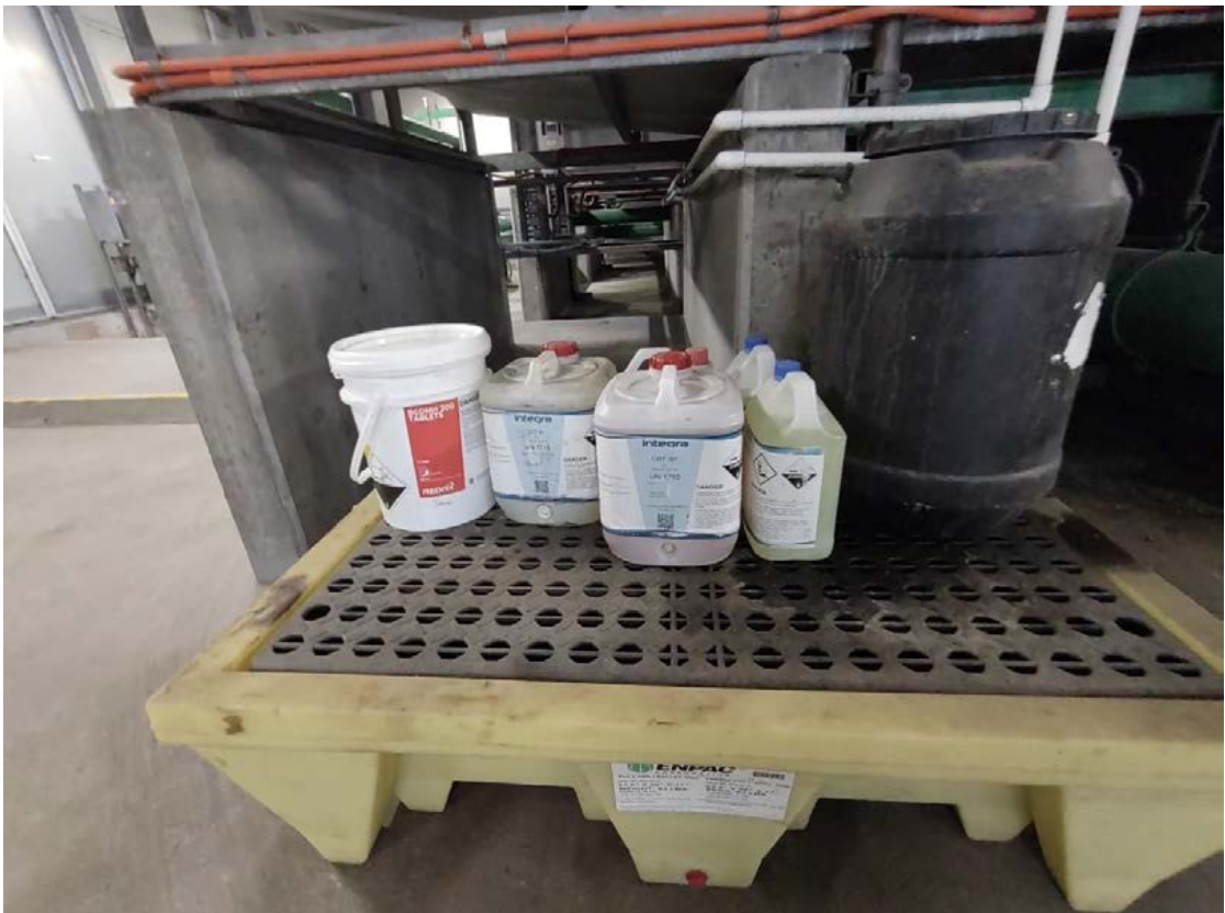
Photo 6: Chemical containers stored in cooling tower room
