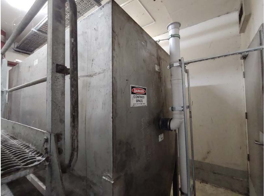
Photo 20: Grease arrester room in basement 2
