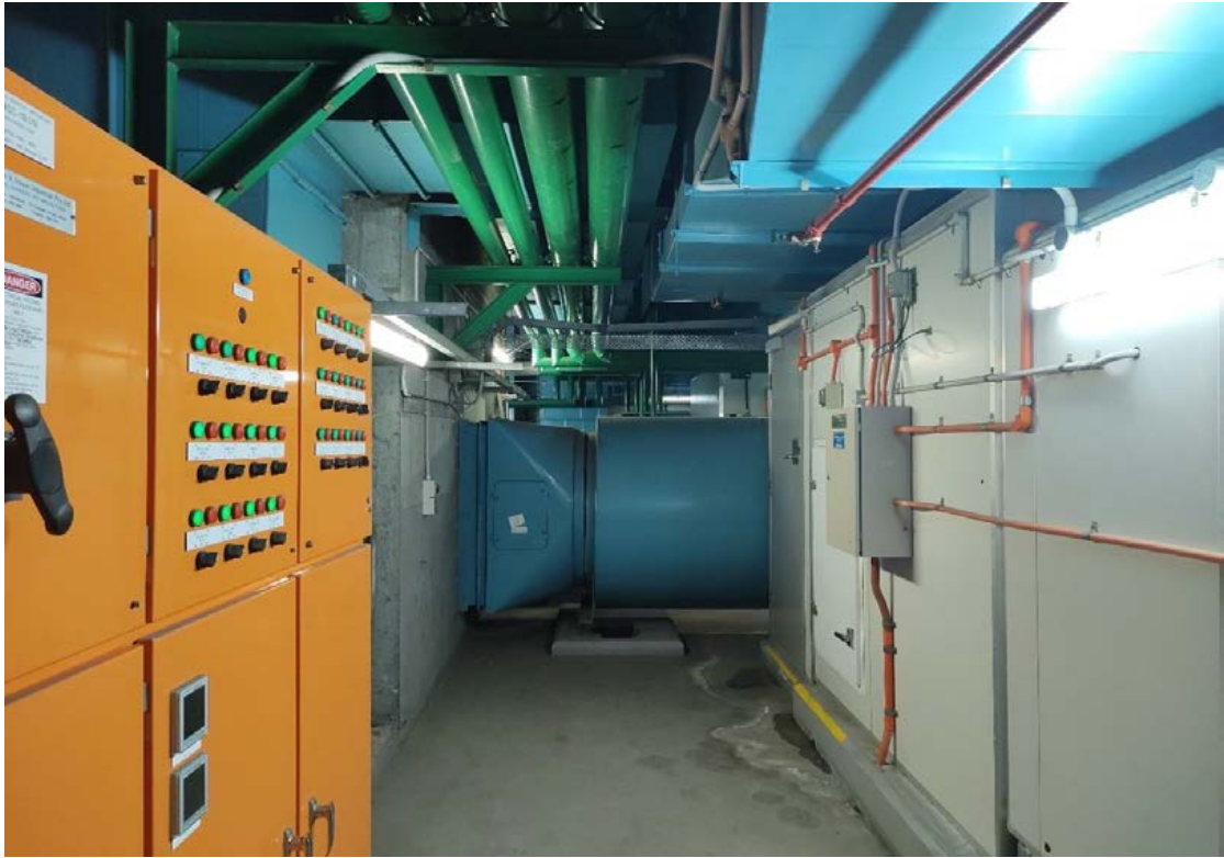
Photo 1: Plant room in level 19
